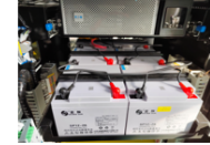
(5) a, Use a red battery jacket to cover the positive electrode of the battery. b, The black battery cover of yoga is placed on the negative electrode of the battery. c, Fix the wire on the battery hoop with a strapping belt and keep the "UPS" and the battery free.
